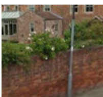
Red brick walls with garden wall bond, hard up to the back of the footpath.
